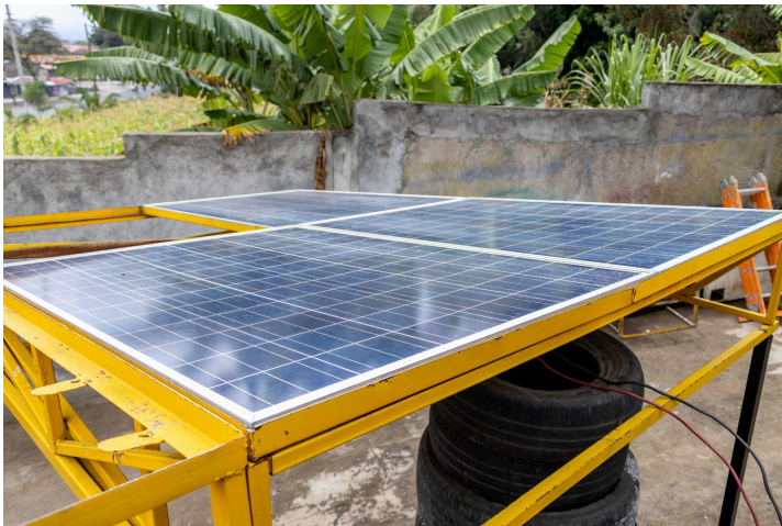
Figure 5: A solar panel structure
