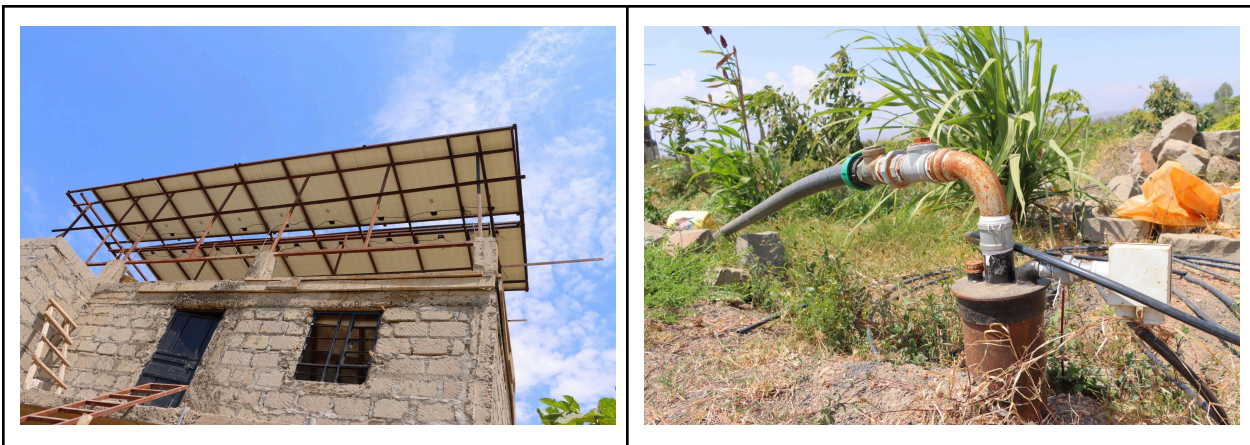
Figure 4: Installed solar-powered irrigation system at George's farm
